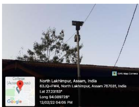
Fig. 10 Solar Street lights installed in the college campus
