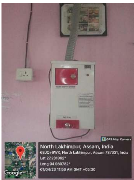
Incinerator 1 at Girl’s Common Room
