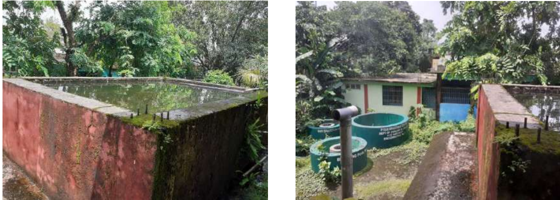
Fig. 11 Rain water harvesting systems in the college campus
