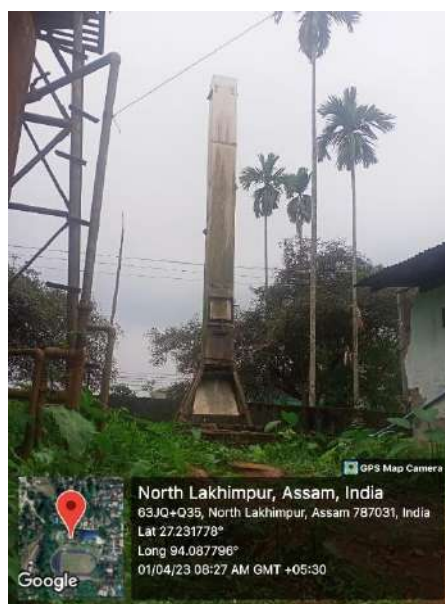
Incinerator 2 at Girl’s Hostel
